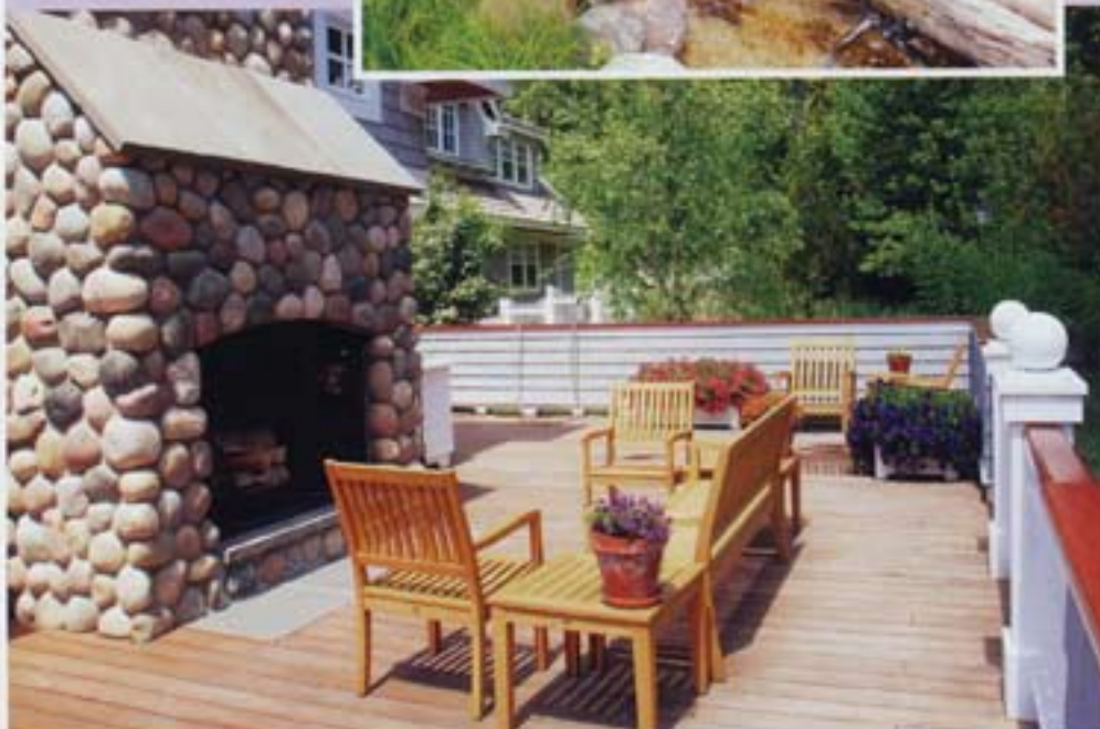
Crews from Dan Hayes Masonry handled the bulk of the stonework inside and out at the property featured here, including five fireplaces and hearths, porch decks, steps and piers. The company also handled the bluestone installation in and around the pool and pool deck.
